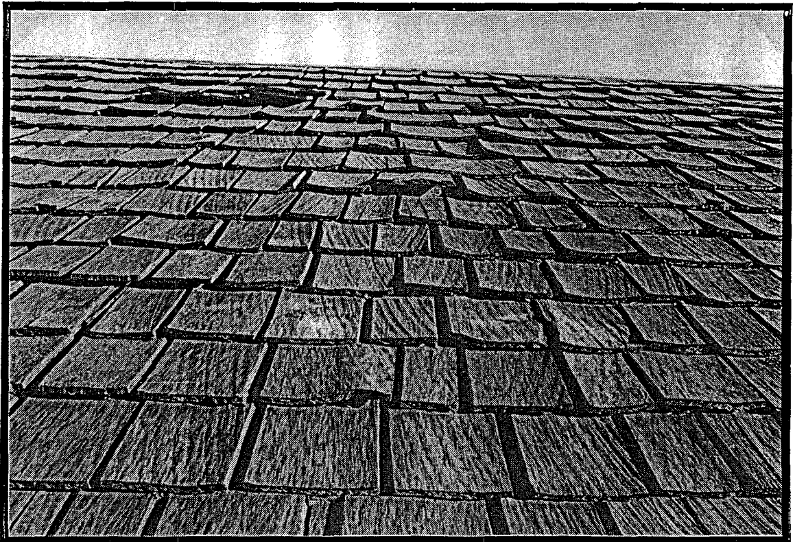
Figure 18. Aspen Test Roof Close-up; Note Various Defect
