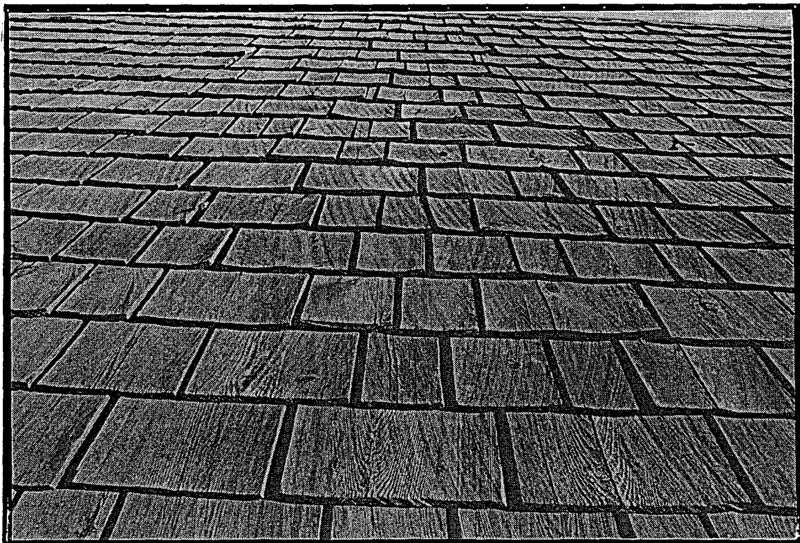
Figure 20. Pine Test Roof Close-up; Note Cracks and Flat Sawn Shingles
