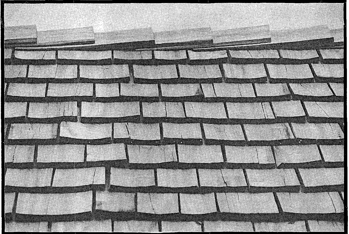
Figure 38. Yellow Poplar Test Roof; 4 Years old; East Texas
