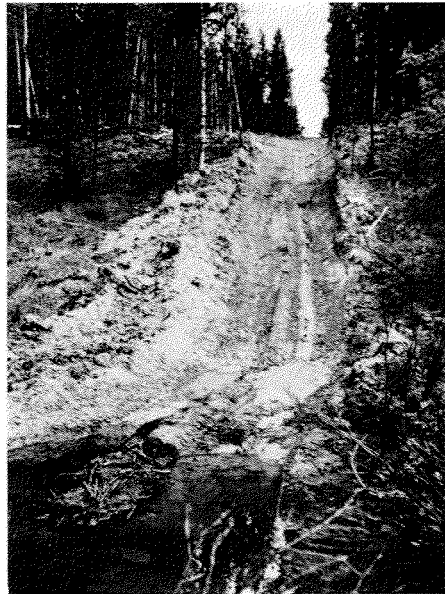
Seismic trail-stream intersection showing severe soil disturbance and sediment deposition at bottom of slope. Most serious sedimentation occurs during periods of high rainfall and streamflow, and during or shortly after road construction when soils are easily eroded and before plant cover can provide protection.
