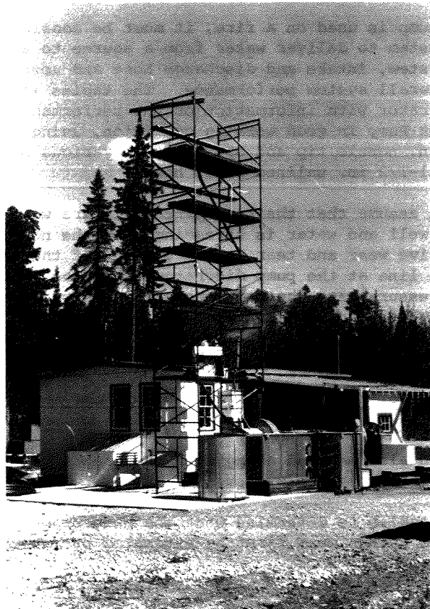
Photo No. 4. Tower for suction lift test.
