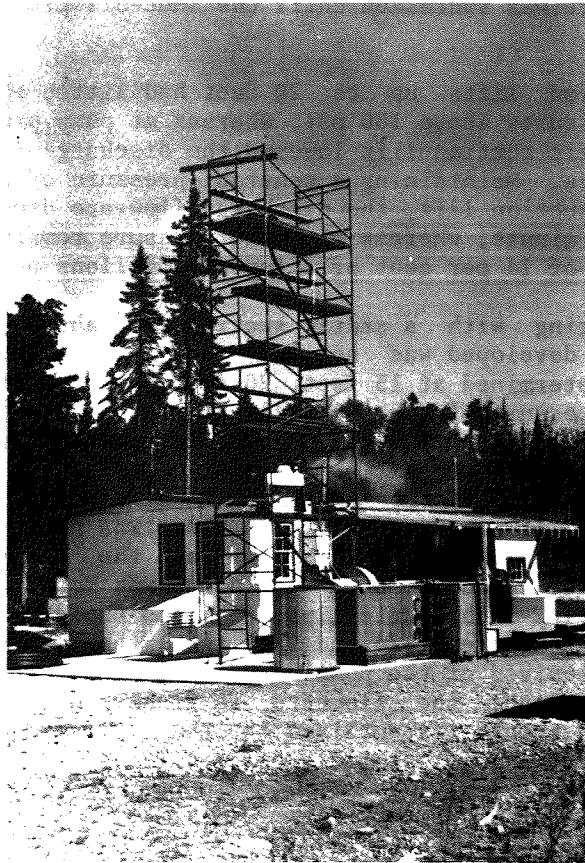
Photo No. 4. Tower for suction lift test.
