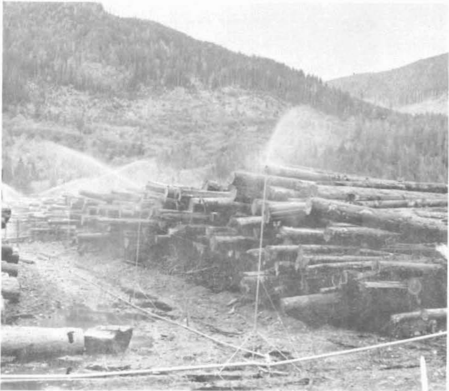
Figure 2. View between log bays shows arrangement of water lines, risers and sprinklers. Note nearby forest, source of attacking beetles.
