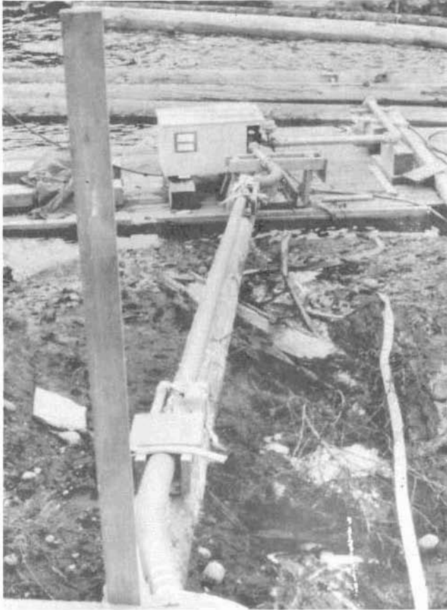
Figure 3. Pump on float, showing two flexible connections to allow for tidal movement.
