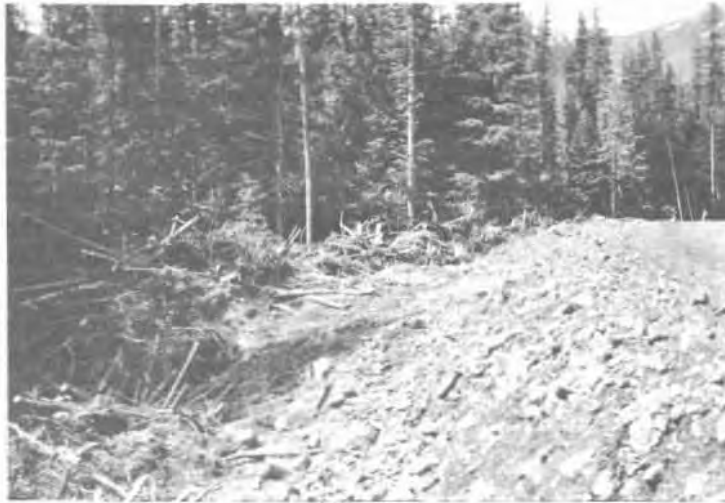
Figure 5 Insufficient fine soil to bury right-of-way debris.
