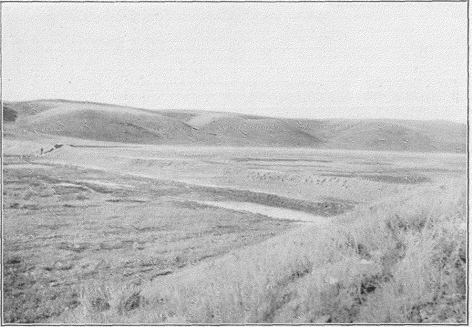
Photo F. T. Fletcher, 1911. Typical Prairie Reservoir under Construction, N. C. Nelson. Tp. 5, Rg. 24, W. 3rd M.
