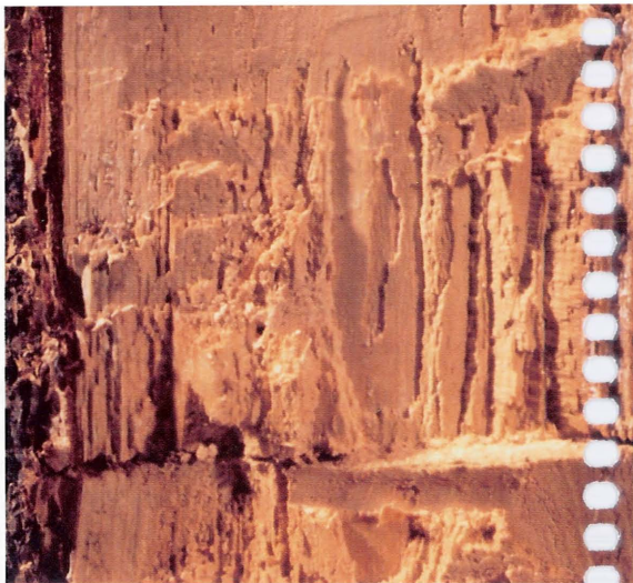
Fig. 44 Brown crumbly rot caused by Fomes pinicola .
