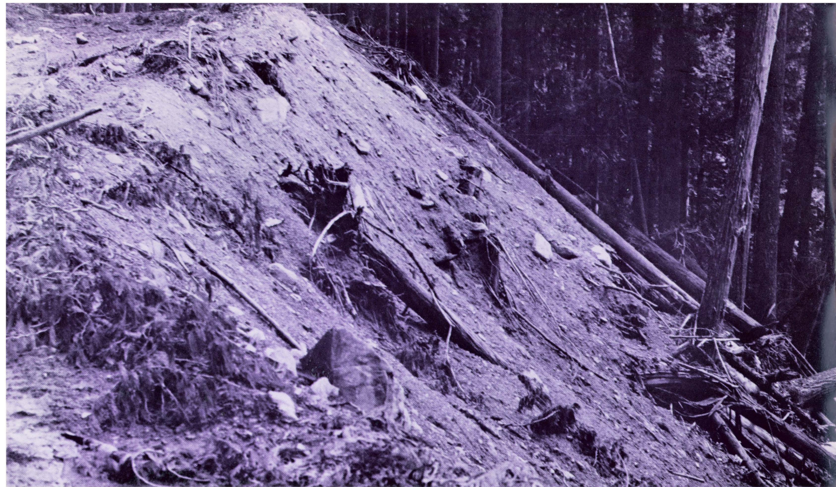
Sidecast material reduces productivity by covering considerable down-slope area with coarse and relatively infertile subsoil and blasted rock.
