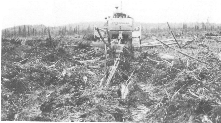
Figure 3. Site preparation for aerial seeding using a modified SIECO fire plow and Michigan floating hitch can produce 30-35% mineral-soil exposure.
