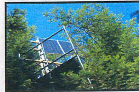
Solar Panels on a Tower
