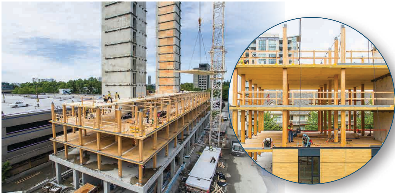
The 18-storey wood building under construction at the University of British Columbia, in Vancouver.
