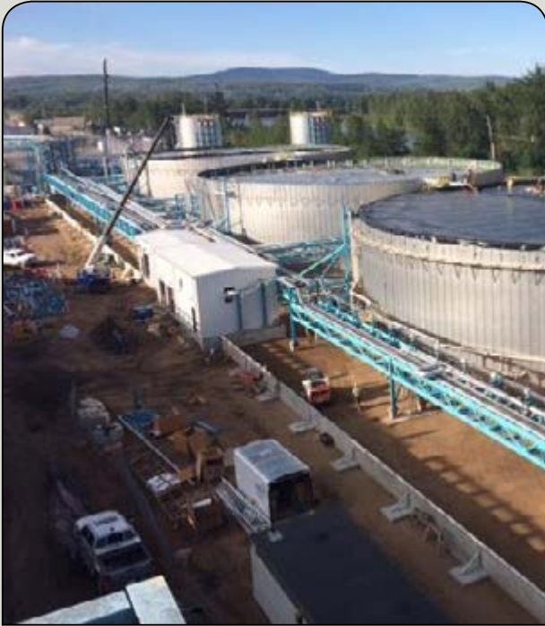
Anaerobic hybrid digester: Anaerobic (no oxygen) treatment uses microorganisms to convert organic matter into biogas from industrial wastewater containing a high concentration of biodegradable organic matter.
