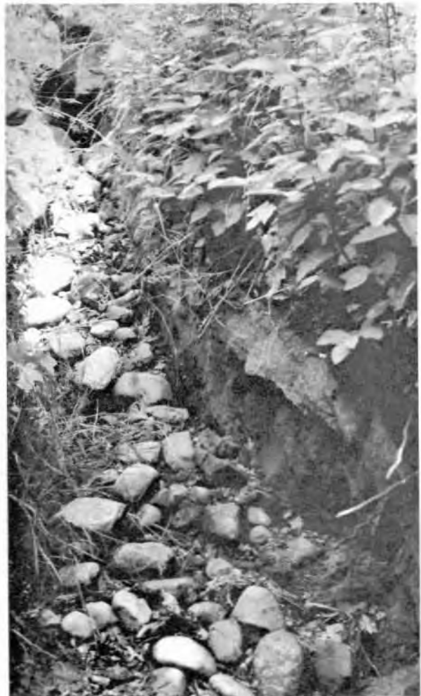
FIGURE 28 - An erosion channel formed where a road crossed the Alluvial Channel Landscape Unit.
