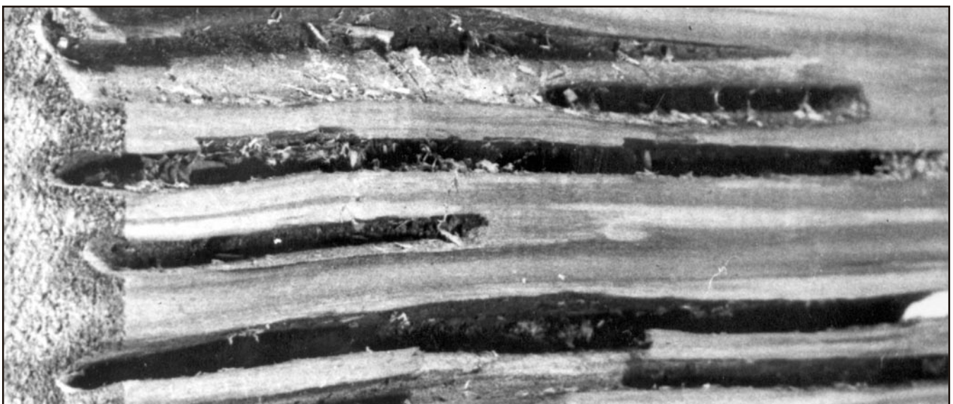
Fig. 5. Carpenter ant damage to a plank.
