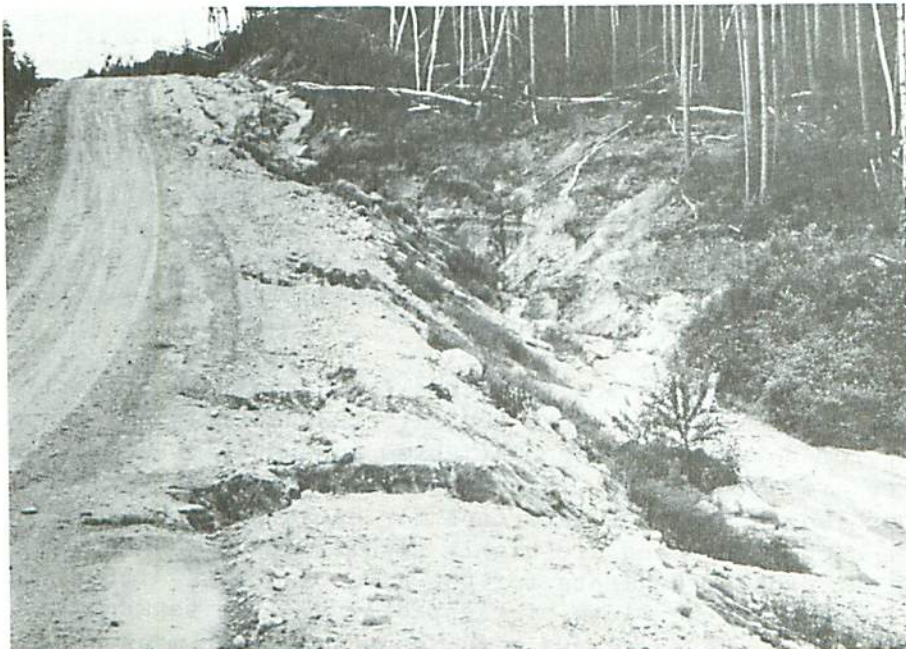
Bank wash and gully erosion (ditch line)
