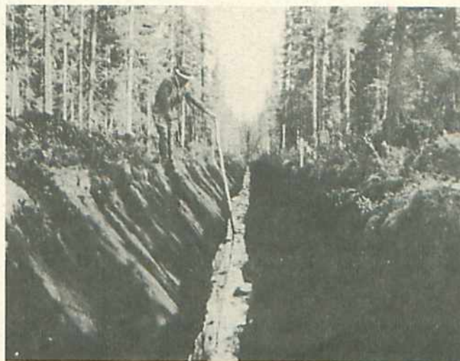
Figure 1. Photograph taken in 1929 shortly after the completion of the drainage ditches near Iroquois Falls, Ontario.
